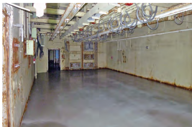
RSL 1 RLOB Sprint Remote control equipment room with ice floor
